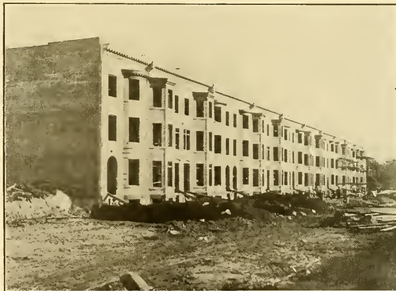
Two-family Houses under Construction by the American Real Estate Company, on Faile Street, in the Hoe Tract
